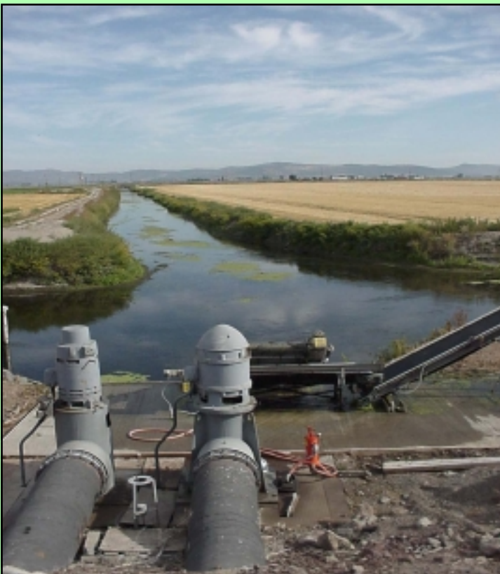
A view of pumps and a delivery canal in the Tule Lake Irrigation District.
