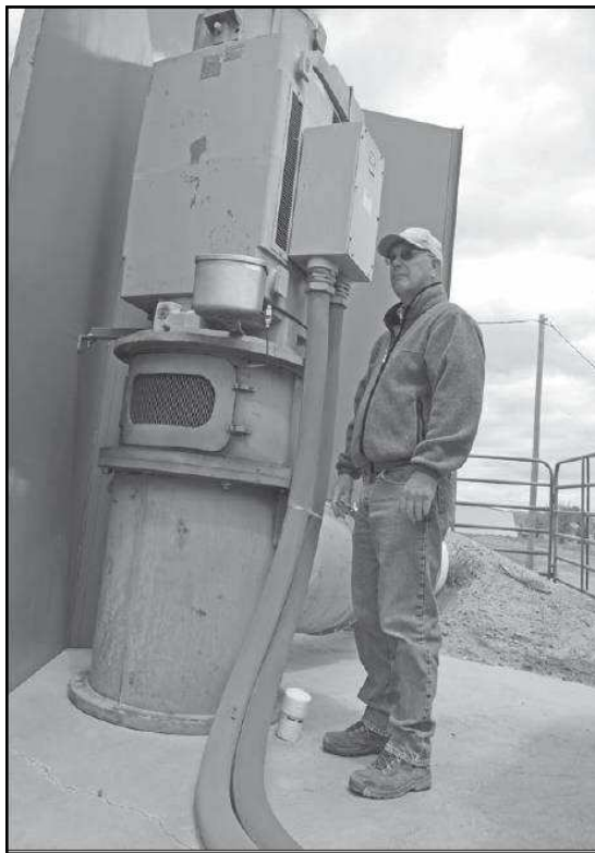
Jerry Pyle stands next to one of the Tulelake Irrigation District wells on the state line. Source: Herald & News
